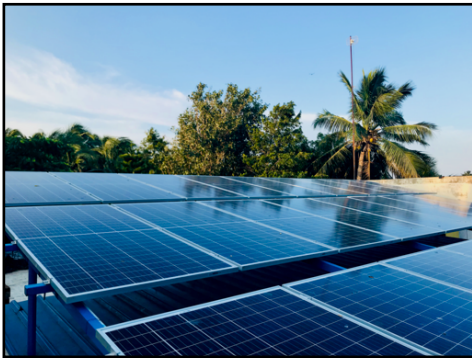
Solar panels on top of the Aum Pranava Building
